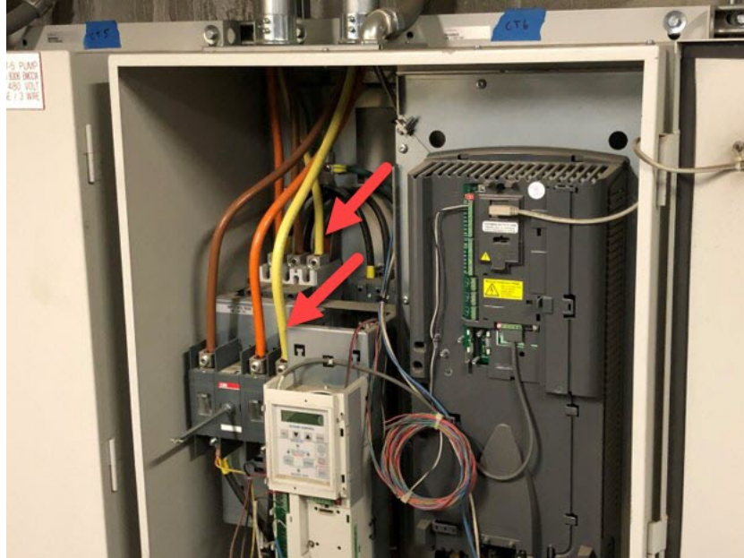
Figure 1: VFD interior with red arrows to loose connections
