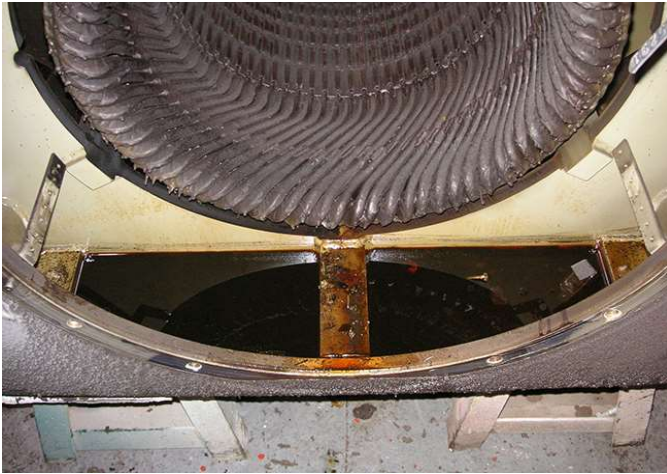
Fig. 5. 800 hp induction motor stator with no missing wedges
