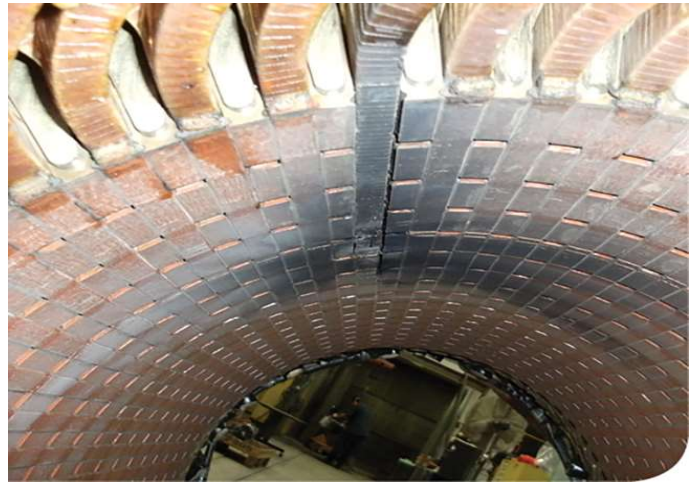
Fig. 7. Stator of DFIG missing wedges and failure point
