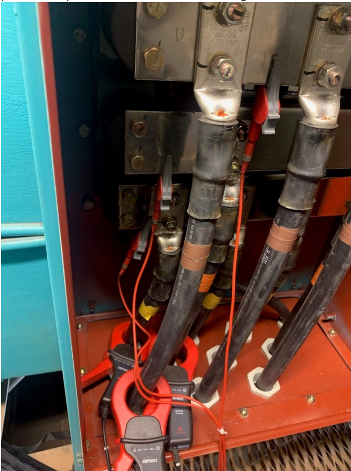
Figure 15: Voltage and current connections at generator. CT ratio used is 3:1 with one clamp around 1/3rd of cables per phase.
