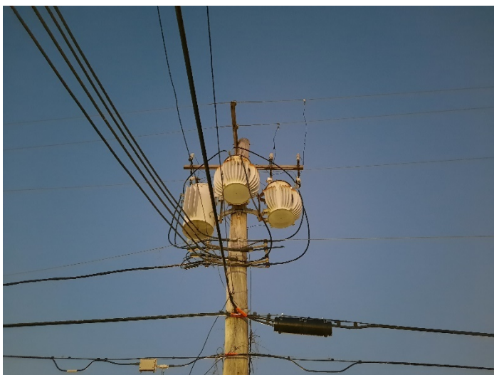
Figure 14: pole mount transformers. The one on the left is Phase 3, middle is Phase 2 and right is Phase 1. Different transformers and resulting unbalanced circuit impedance plus possible loading at the neighboring facility.
