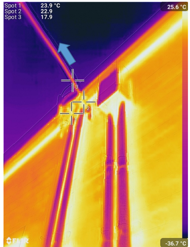
Figure 11: IR of line coming to the outside disconnect of the facility.
