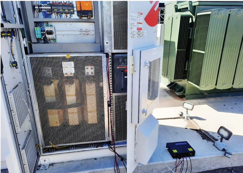
Figure 9: Solar Transformer Being Tested and Evaluated between Primaries from the Output of the Solar Inverter
