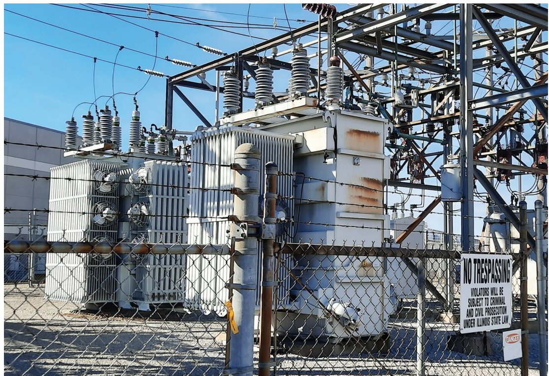
Figure 1: Oil-Filled Transformers with Bushings (top), Fins, and Fans
