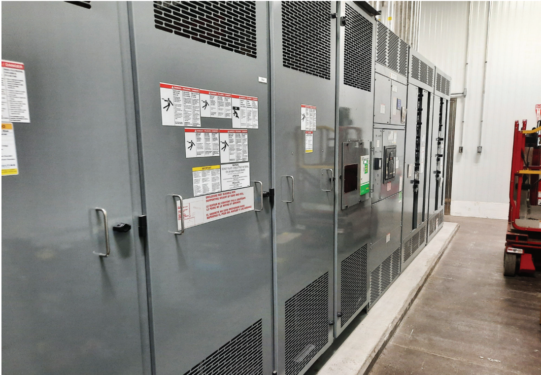
Figure 2: Dry-Type Transformer with Vents at Top and Bottom Internal fans operate to cool the transformer.
