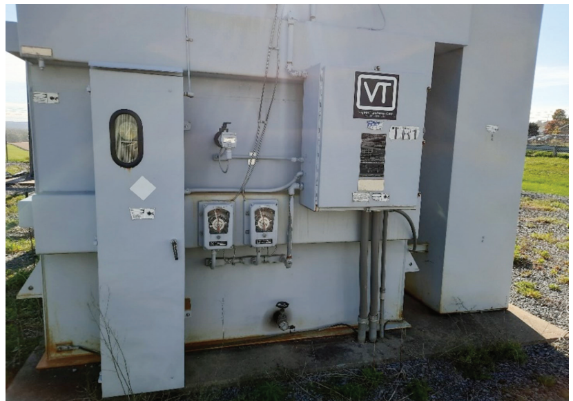
Figure 3: 125 kV to 13.8 kV Transformer with Low Power Factor and High Harmonic Loads
